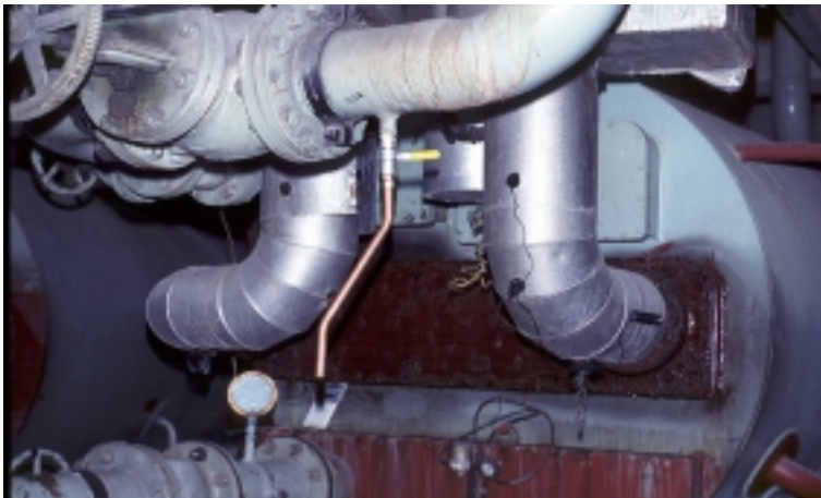
Sampling point on cooling water return pipe courtesy of Dr John Lee
